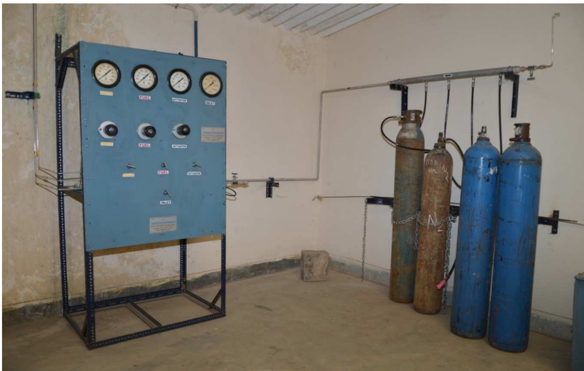
Control panel and high pressurization system for fuel and oxidizer tanks
