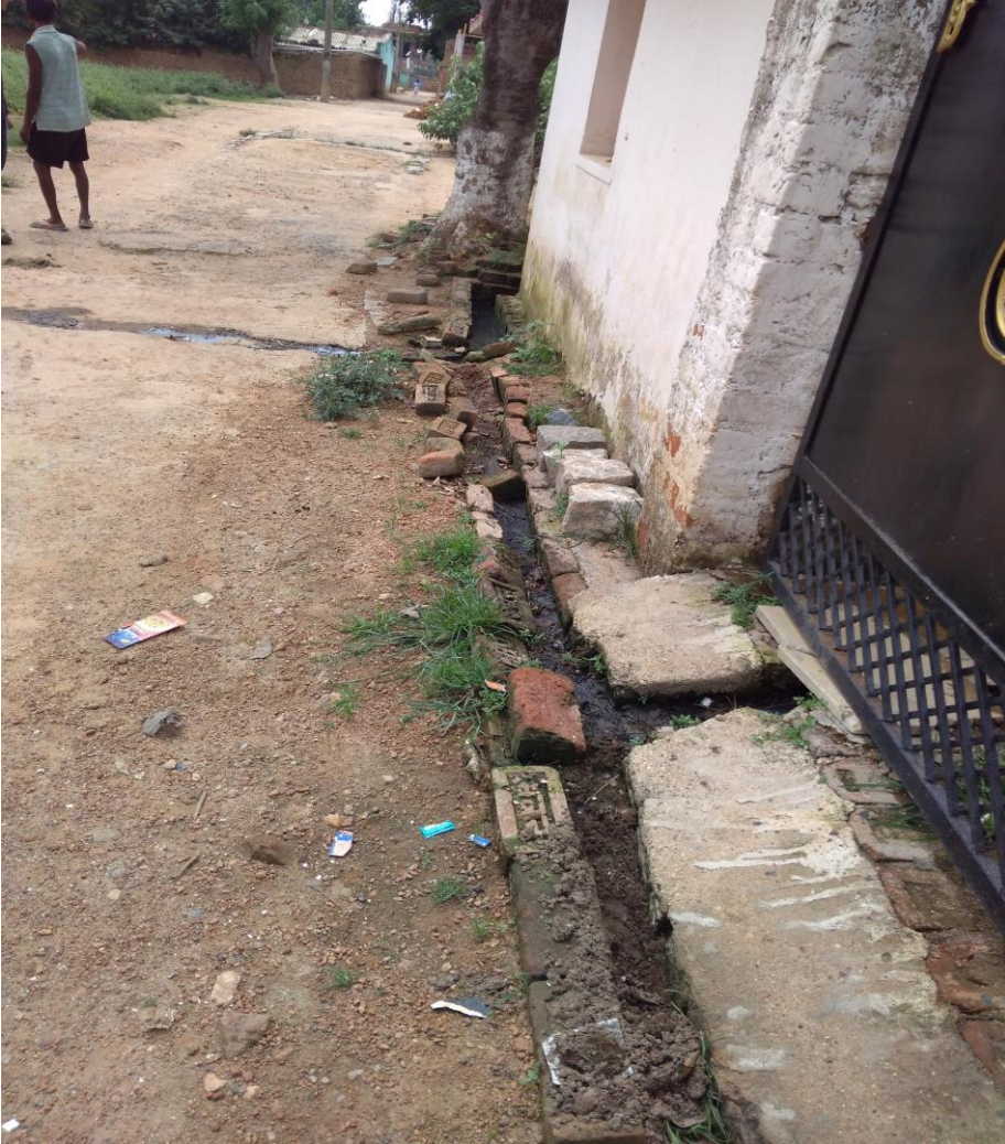
The Present Drainage Condition at Entrance
