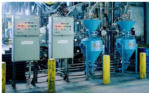
A brief glimpse of pneumatic conveying systems
