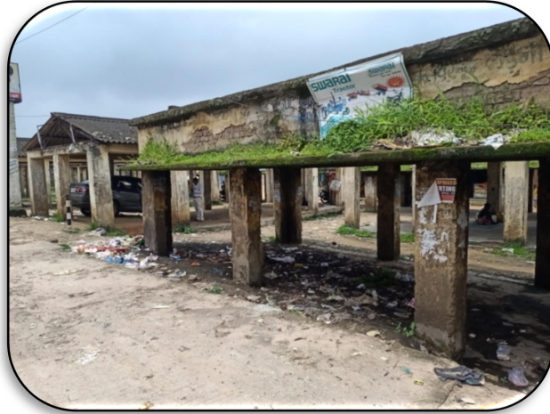
Fig. 4.6: Rural Haat (Weekly Market) along roadside near Vikas Chowk in dilapidated condition
