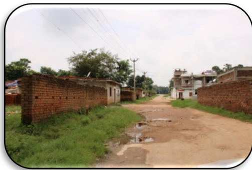
Fig. 7.12: PCC roads which needs maintenance
